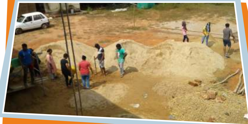
Volunteering for Construction of School Building at D.K.Z.P Higher Primary School, Daddalkadu
